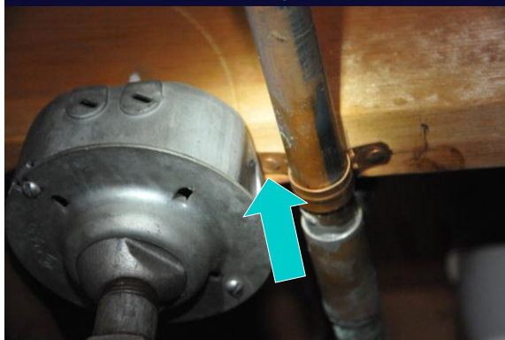
The pipe bracket is contacting the junction box
