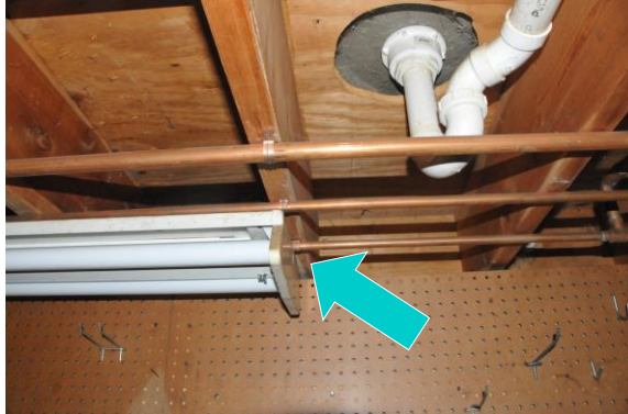
The fluorescent light fixture is in contact with the pipes
