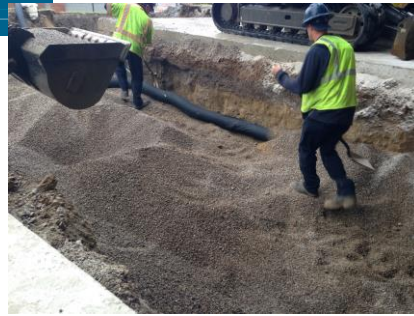
Buried perforated injection piping
