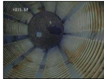
• Various pieces of debris identified at the bottom of a casing
