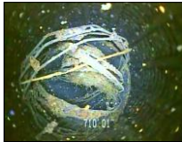
• A wire obstruction located at 710 feet
