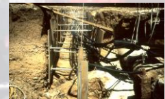
Contractor supported these communication lines by placing timbers across the trench then using strapping.
