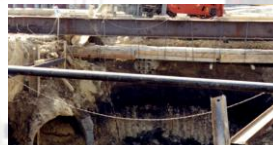
An "4" beam and chains were used to support the concrete "duct-bank" crossing this excavation from left-to-right.
