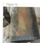
A carbide-studded casing shoe is welded to the bottom of the first casing pipe.
